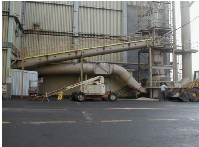
Figure 15. Duraflake's dry storage dust control
